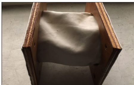
Nicholson's, our organ contractors, have replaced the defective part, so it should give many more years of service. Photos courtesy of Nicholson's.
