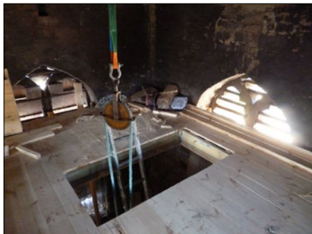
Above the new floor. The arches will remain open, letting the sound of the bells out when the trap-door is open. Photos: David Kelly / Keltek Trust.
